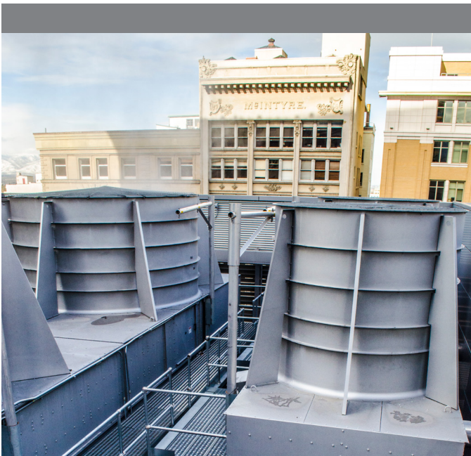
Cooling towers in the City Creek development in downtown Salt Lake City utilize some of the most energy efficient technologies. Photo Credit: Andrew Gillman
