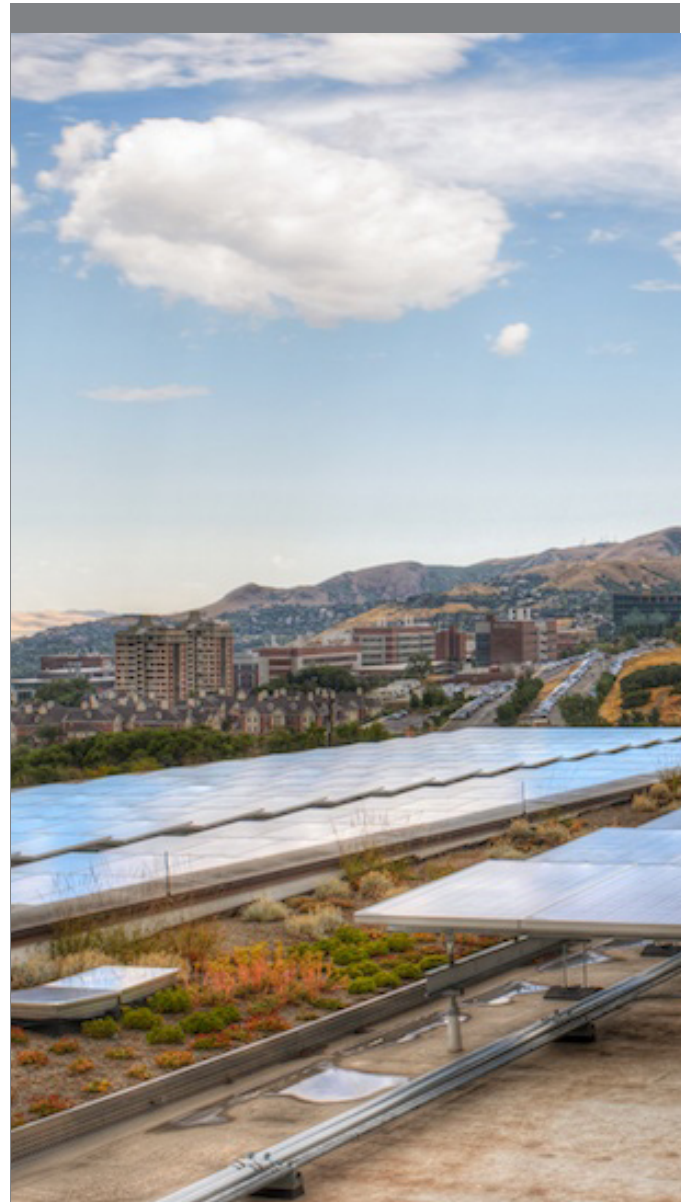
Solar panel installation on the new Utah Natural History Museum rooftop. OED was instrumental in procuring funding for the new panels.
