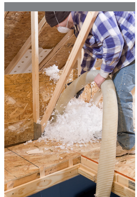
Insulation being blown into attic to increase heat retention in a home.
