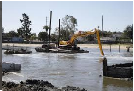
Photo 6: Dredging in the Western Arm; over 70,000 cubic feet of dredge material were removed from the Lagoon and transported to the Port of Long Beach for use in their Middle Harbor project (Pirazzi)
