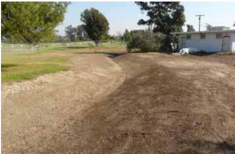
Photo 4: Newly contoured bioswale on the north bank of the Western Arm prior to planting (Zahn)
