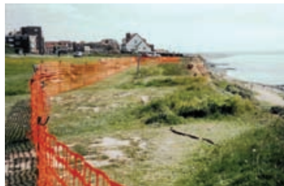
Figure 8. Effects of coastal erosion can affect homes and property as illustrated by the landslide of 18 May 2008, Hoskin's West, Barton-on-Sea, UK (Courtesy Mrs. Page)
