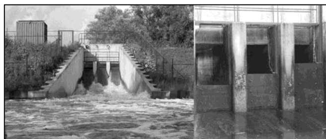
Figure 7. left: inlet structure seen from the FCA side; right: close up of the culverts and the wooden log weirs (photo: [10]).
