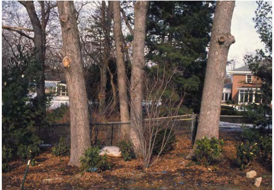
These mature oak trees in a suburban Chicago garden were damaged when major roots were cut to allow the planting of large shrubs close beneath them.
