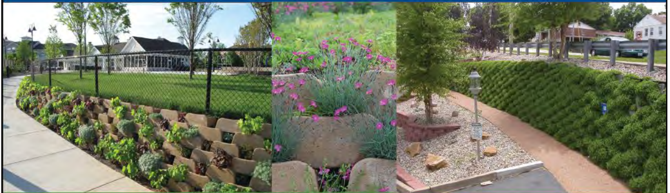
Vertical Gardens/Vegetated Retaining Walls
