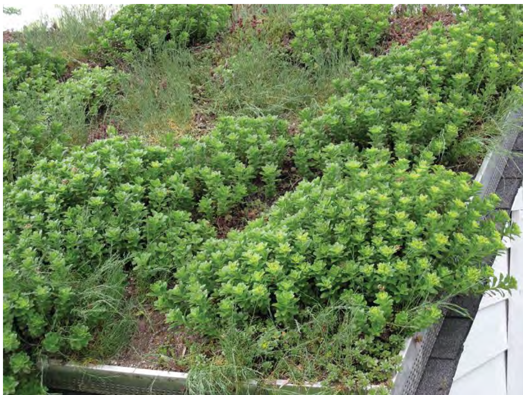
Green or living roofs, such as this one at the AHS's River Farm headquarters in Alexandria, Virginia, can help reduce runoff by absorbing some rainfall in the growing medium.
