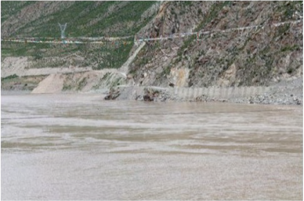
Fig. 5. Stream bank degradation caused by road construction along the Tongtian River.
