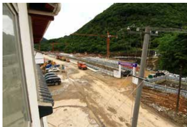
Fig. 17. View of Downtown Pingqian in June 2014, covering same view (different angle) as Figure 16. Photo by Kevin R. Messenger.
