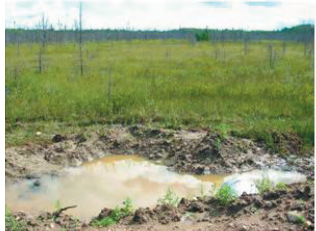
Ineffective installation of culvert under road at Clyde Fen Photo Derek Johnson
