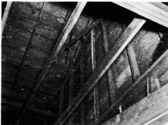
FIGURE 126. Broken studs in north gable, Barracks 2 after Test 2
