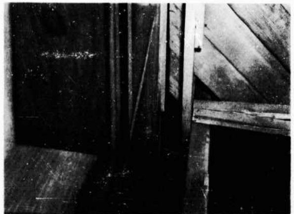
FIGURE 121. Looking up from ground floor, showing separation of south wall from 2nd floor framing, Barracks 1 after Test 2
