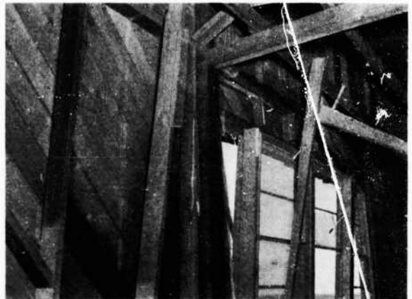
FIGURE 127. Broken and displaced studs, north wall, second story, Barracks 2 after Test 2
