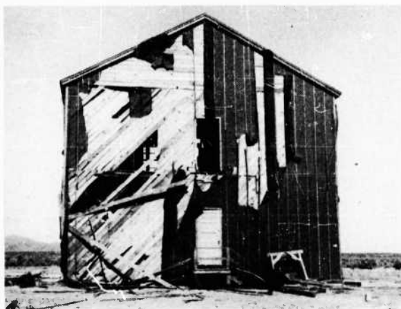
FIGURE 207. South elevation of Barracks 1 after Test 5
