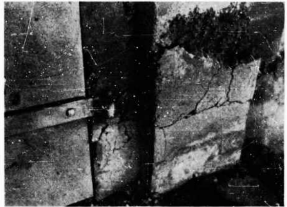
FIGURE 100. Close-up of lower door hinge and pilaster, showing fractured concrete over hinge anchor; Igloo F after Test 2
