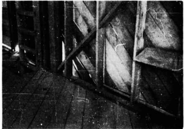
FIGURE 166. Interior, Barracks 1 after Test 3, illustrating displacement of south wall at second floor level
