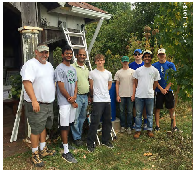
The rain barrel installation crew: (left to right) Jeff Floyd, Pranay Mupparaju, Peter D'Souza, Isaac Tonges, Nicholas Crowe, Eric Witt, Isaac D'Souza and Carter Crowe.
