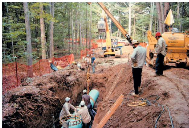
Using a crane with a side-boom, which could hoist from the side instead of the front, meant that the heavy equipment could install pipe in a tighter area without three-point turns, thus limiting the disruption zone.
