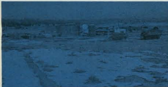
(Below) NEW PLANT SITE — Fairchild's new Shiprock plant, scheduled to be ready this summer, looked like this in February. Construction is progressing on schedule to accommodate the fast-growing facility.
