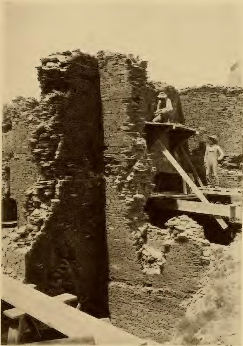
FIG. 116.—Repairing third-story walls in Pueblo Bonito. Some of these high walls had been so weakened by vandalism and the elements that their repair was necessary before excavation could safely be undertaken beneath. The work will serve, also, to preserve the present height of the walls for many years to come. (Photograph by O. C. Havens. Courtesy of the National Geographic Society.)
