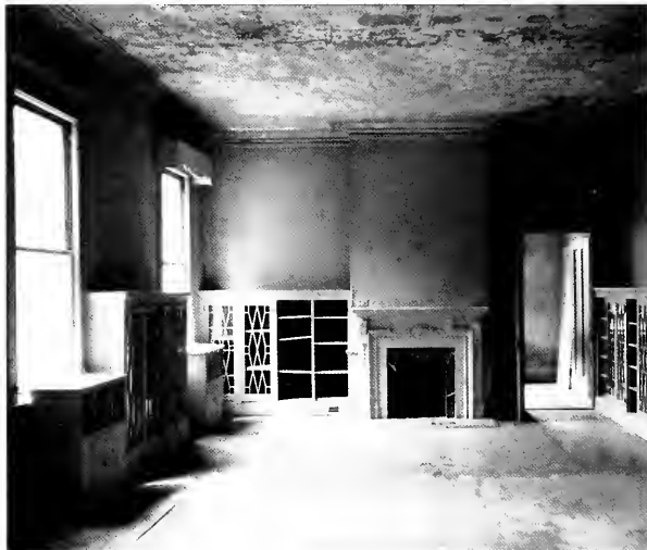
Sitting vacant for two decades, Wise House deteriorated. Inlaid hardwood floors were worn, and plaster on the walls and ceilings was damaged as were the glassed-doored wall cases in the grand room and fireplaces throughout the house.
