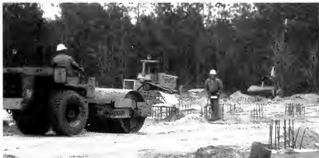
Workers with Clancy and Theys are laying the foundation for UNCW's Science Building
