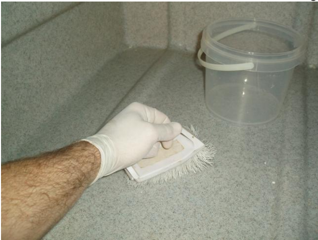
Scrubbing Enclosure (C.Morris09)
