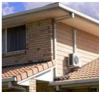
Air-conditioning unit visible
