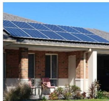
Photovoltaic panel facing street
