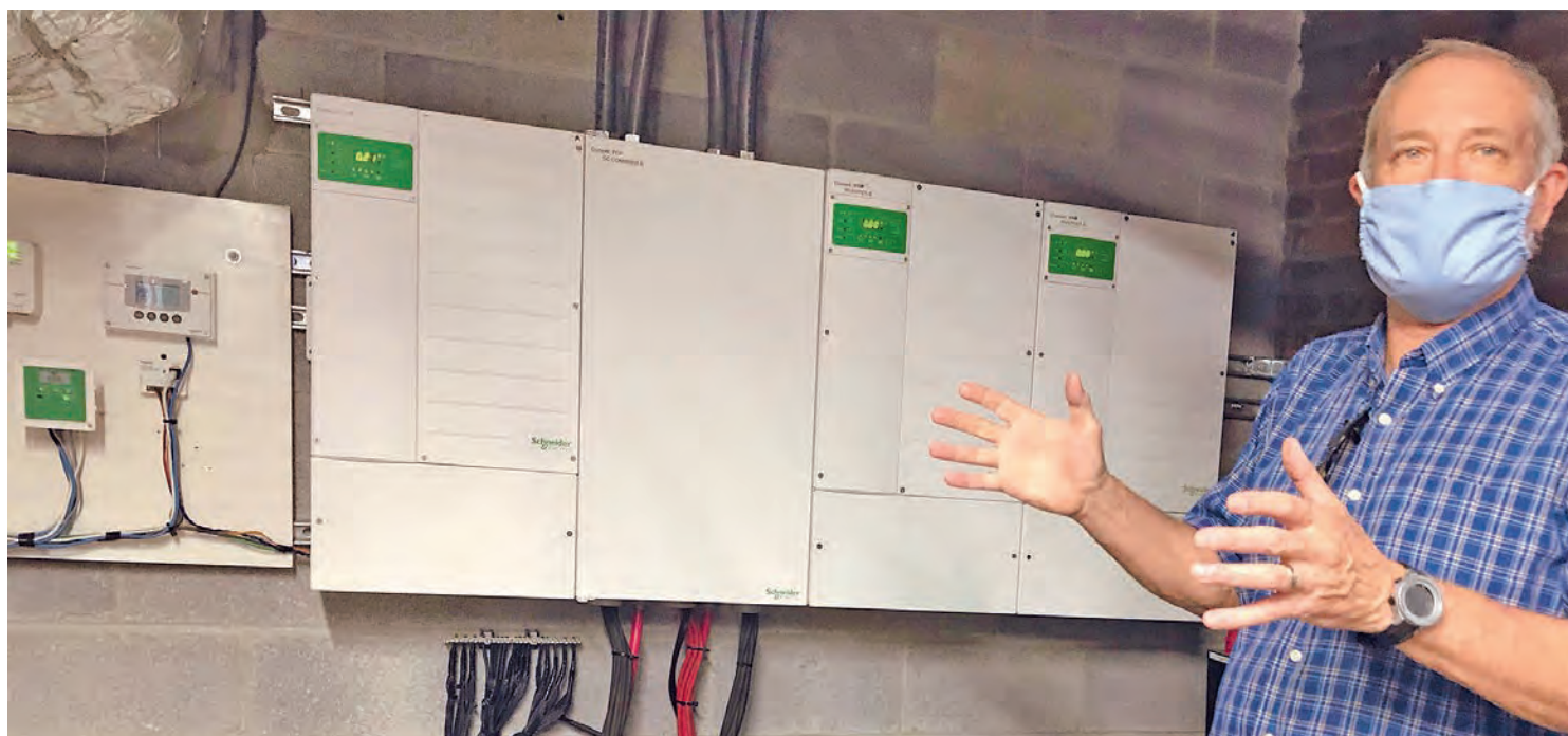
Martin Mellett, vice president for external affairs of Jubilee Housing, explains how in a power blackout, backup batteries installed at the Maycroft Apartments can provide power for up to three days to the building’s Teen Center, a learning, recreation and meeting space which in such emergencies doubles as a “resiliency center.” Solar panels on the four-story building’s rooftop recharge the batteries. (Timothy B. Wheeler)
