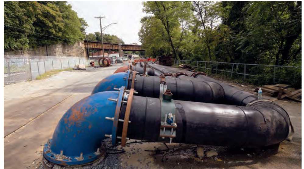
Under a consent decree to fix chronic sewage overflows, Baltimore city requested extensions because of the pandemic on its mandated schedule for making sewer repairs like this one along the Jones Falls. The state denied them. (Dave Harp)
