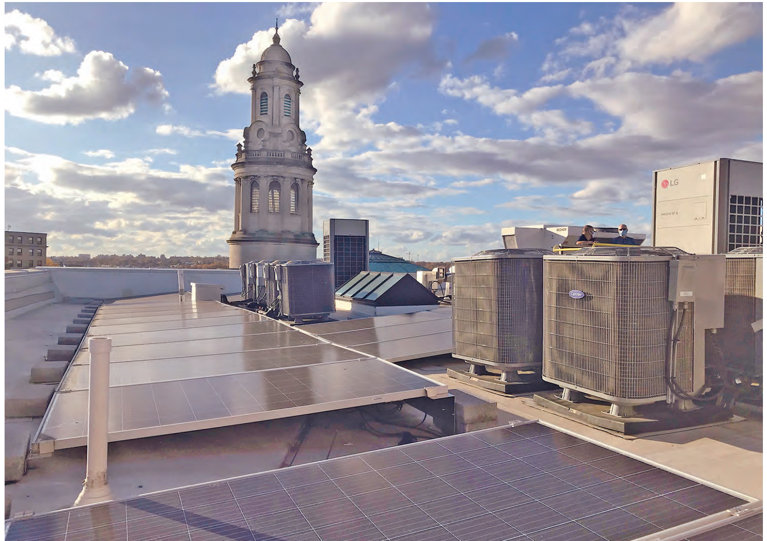
The rooftop of the Maycroft Apartments in the District's Columbia Heights neighborhood is covered with 192 photovoltaic panels, squeezed in among air conditioning units, skylights and vents. Electricity generated by the solar array goes to the grid, earning the building's residents sizable credits on their power bills. (Timothy B. Wheeler)
