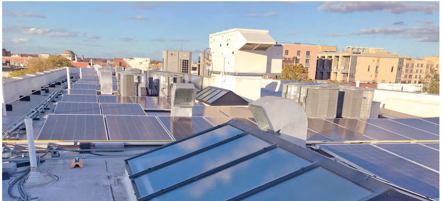
Solar panels that make use of rooftops, like these on the Maycroft Apartments in the District's Columbia Heights neighborhood, can both protect waterways and achieve clean energy goals. (Timothy B. Wheeler)
