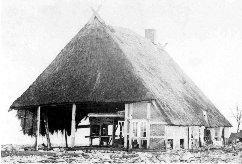
Figure 1. Destroyed building in Niendorf at the Baltic Sea coast after the storm surge of 1872 (Source: Gemeindecarchiv Timmendorfer Strand).
