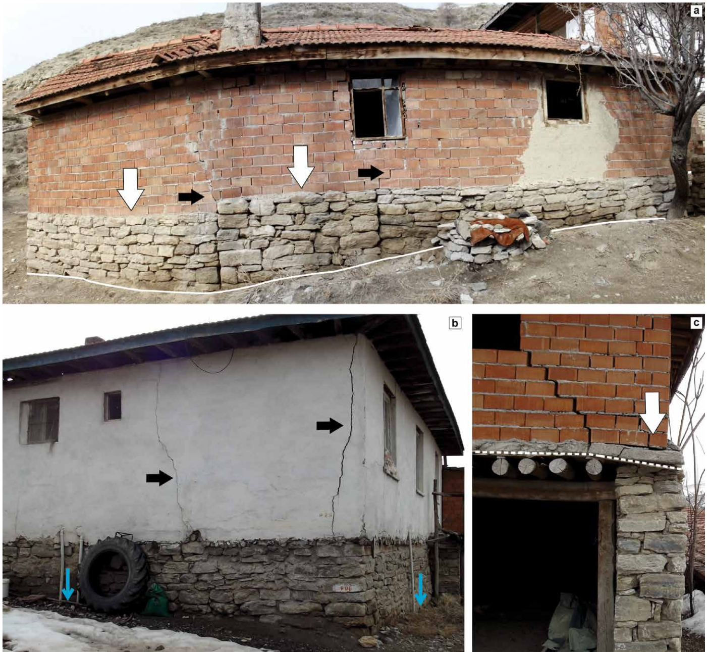
Figure 4. (a) Displacement of house wall showing bulging and cracking caused by subsidence, and broken windows due to distortion. (b) Cracks on wall and pipes draining wastewater directly into ground. (c) Open joint in wall of building. (Photographs taken on February 26, 2017).
