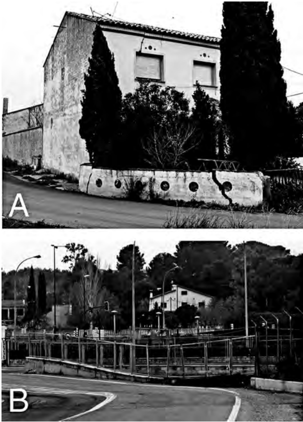
Figure 4. Damage in urban areas northwest of the city of Zaragoza resulting from karst subsidence. A, fractures in walls. B, strong deformation of a fence.
