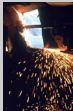
Large access holes were cut throughout the ship to allow for current flow and to increase diver safety.
