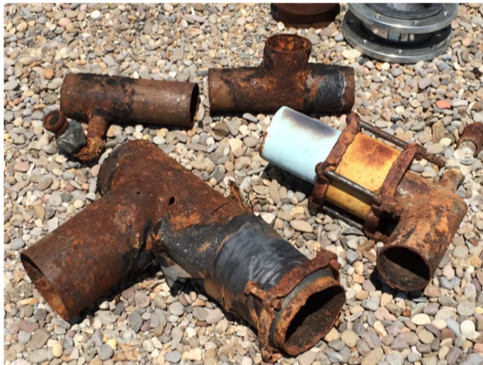
Photo 3-4 Typical Failed Pipes
