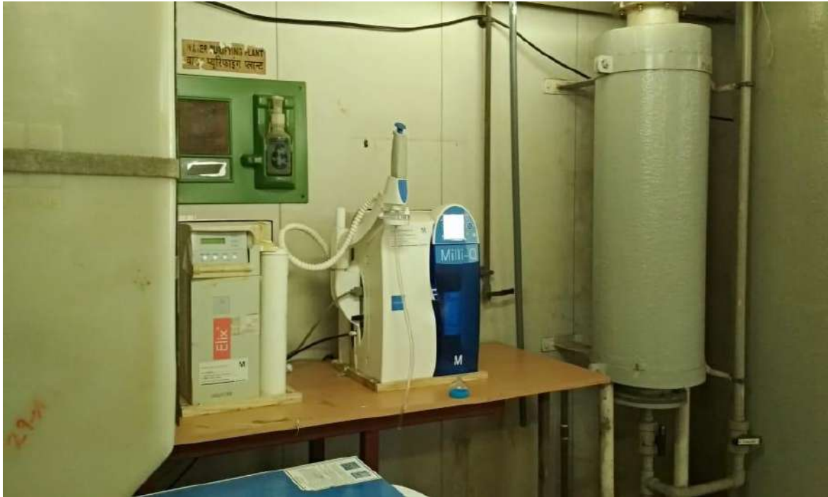
Water purification plant (Wet lab)
