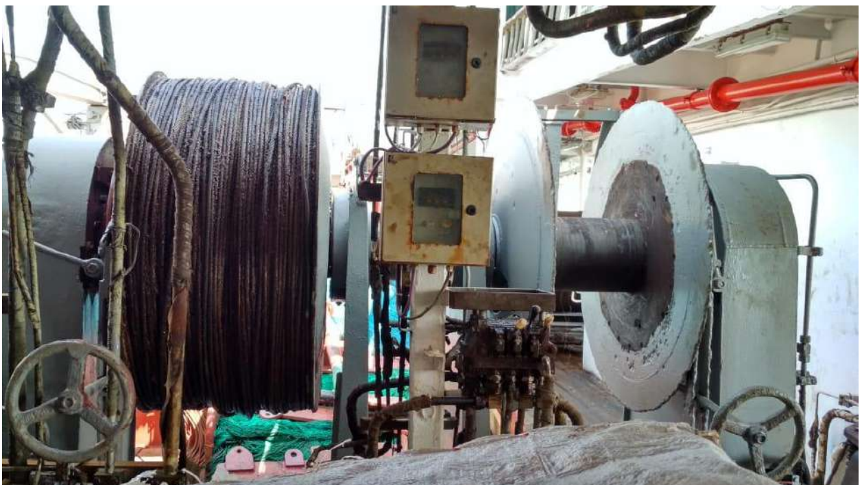
Sweep Trawl winch – for Dredge operation.
