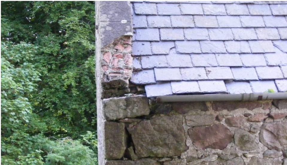
Photo 9: Southeast corner of building. Damage to wall and a missing slate has caused a large crack to form. This has no bat roosting potential and no evidence of bats was found.
