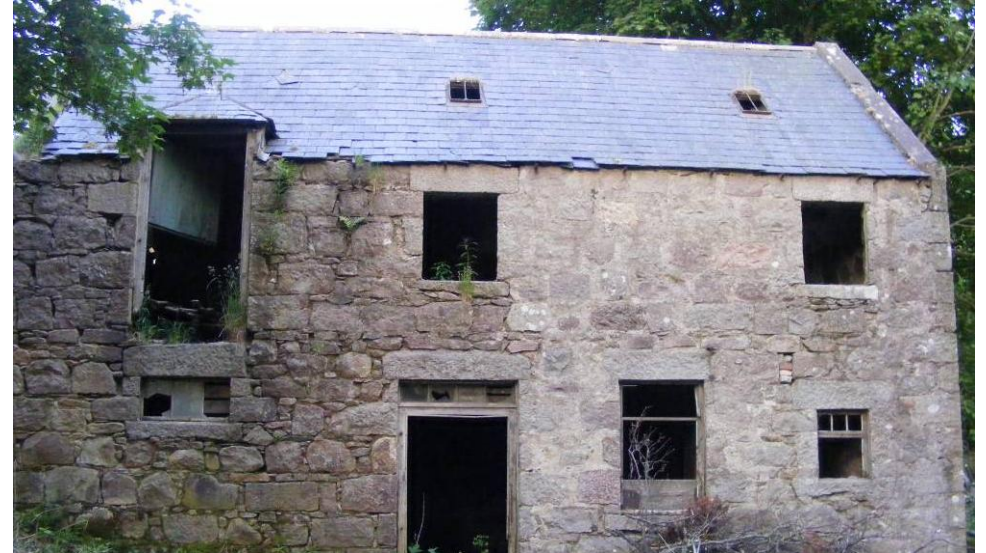
Photo 5: West elevation of mill. Plants are growing from cracks in places show wall is damp. Some loose and missing slates on roof provide limited bat roost potential. No evidence of bats found.
