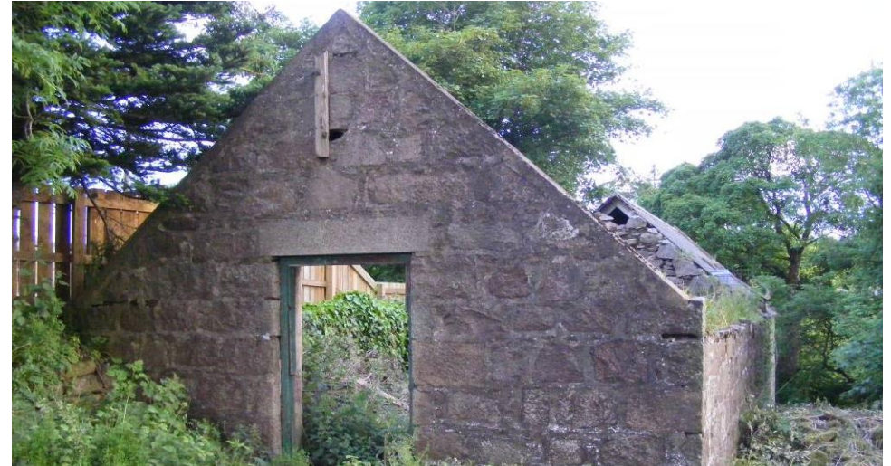
Photo 1: North gable of ruin. In good condition other than large crack next to wooden board. No evidence of bats.
