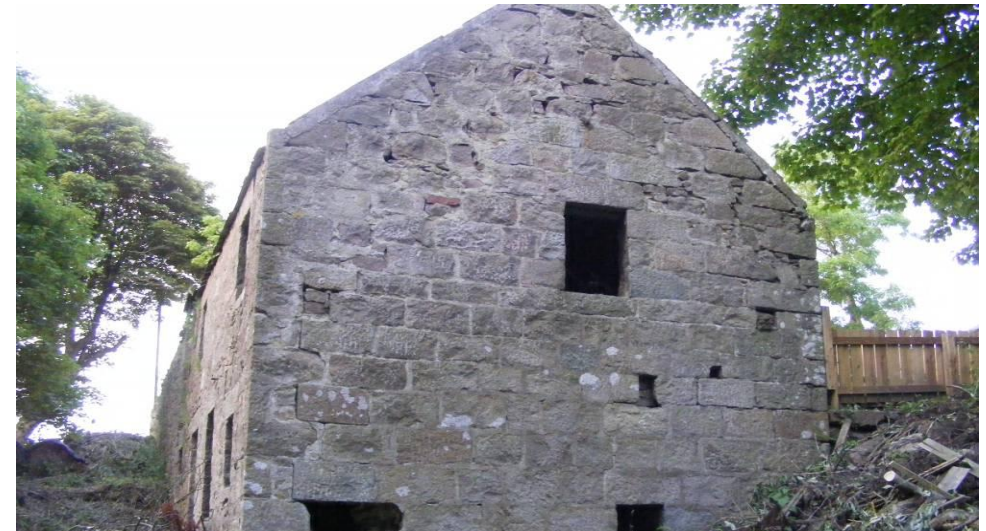
Photo 7: South elevation of mill. Some large holes in wall which had some cracks, however, no evidence of bats were found. Small, shallow cracks near top of mill could provide limited roosting potential. No evidence of bats was found.
