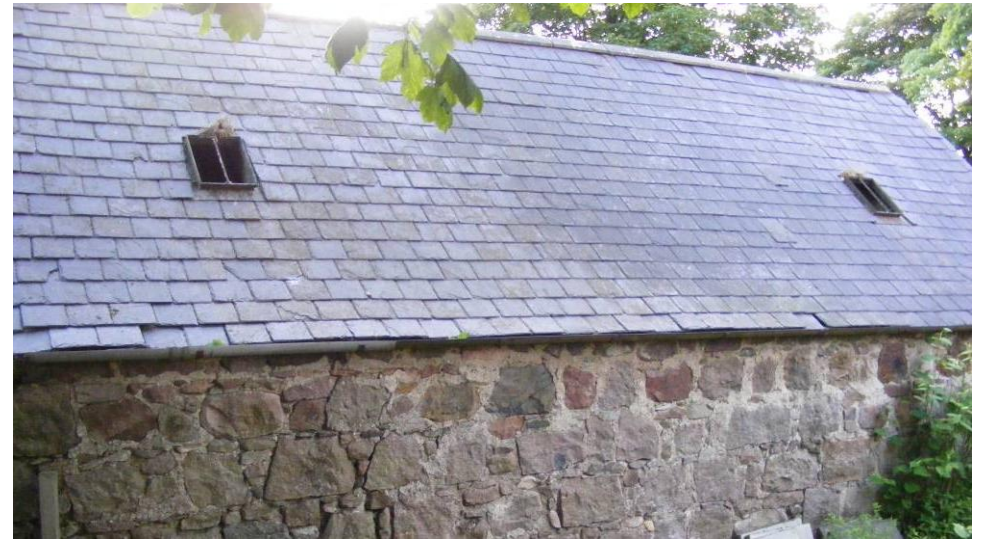
Photo 10: Eastern elevation of Mill building. Roof has several missing slates but is mainly in good condition. Windows are broken allowing water inside contributing to the damp. Ridge appears intact.
