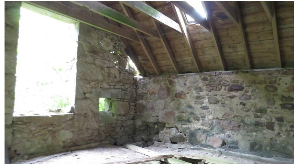
Photo 11: North gable. Large hole in northeast corner of the wall. Roof and floor rotten in places. The building is in poor condition and becoming dangerous.
