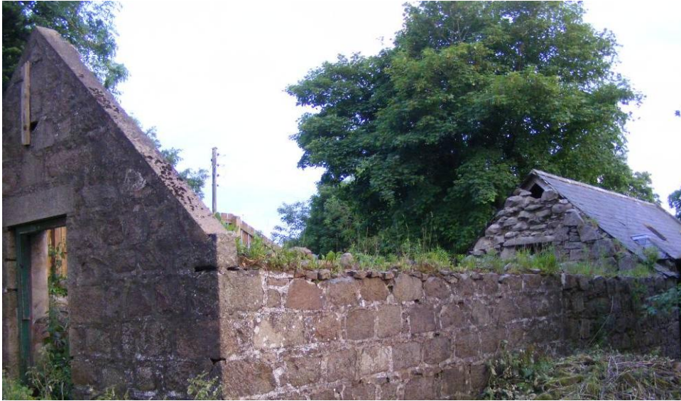
Photo 3: Northwest corner of ruin. Remaining wall generally well-sealed.
