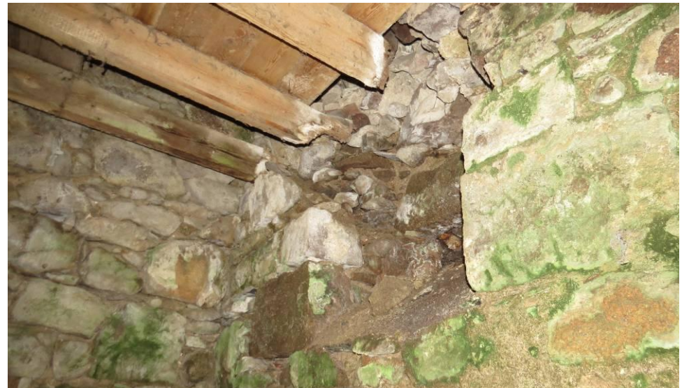
Photo 15: Lower floor ceiling beams rotten and dangerous. The wall is very damp with no bat roost potential.
