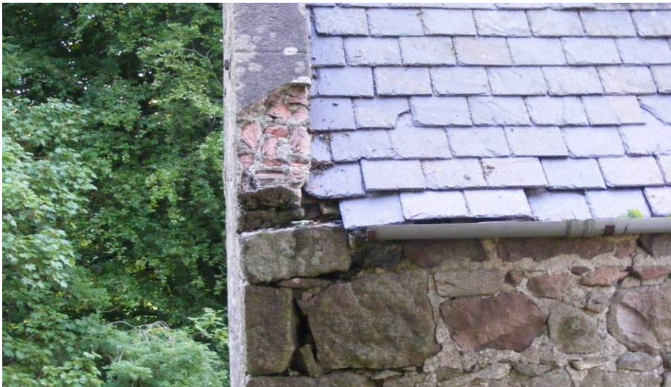
Photo 9: Southeast corner of building. Damage to wall and a missing slate has caused a large crack to form. This has no bat roosting potential and no evidence of bats was found.
