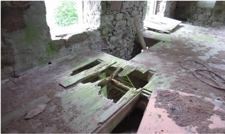
Photo 12: View of staircase from ground floor to lower ground floor. Area is dangerous with rotten floorboards and some joists are not attached to the wall.
