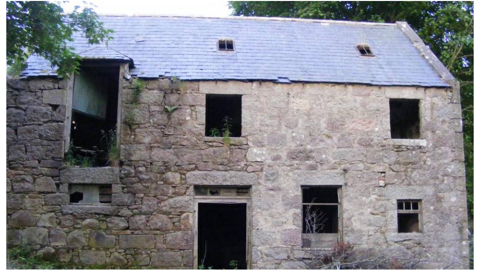
Photo 5: West elevation of mill. Plants are growing from cracks in places show wall is damp. Some loose and missing slates on roof provide limited bat roost potential. No evidence of bats found.
