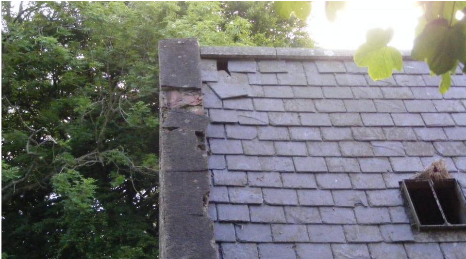
Photo 8: South gable end. A loose slate has caused a small hole in the roof contributing to the dampness inside the mill and in the roof. Lifted and missing slates provide limited roosting potential. No evidence of bats was found.
