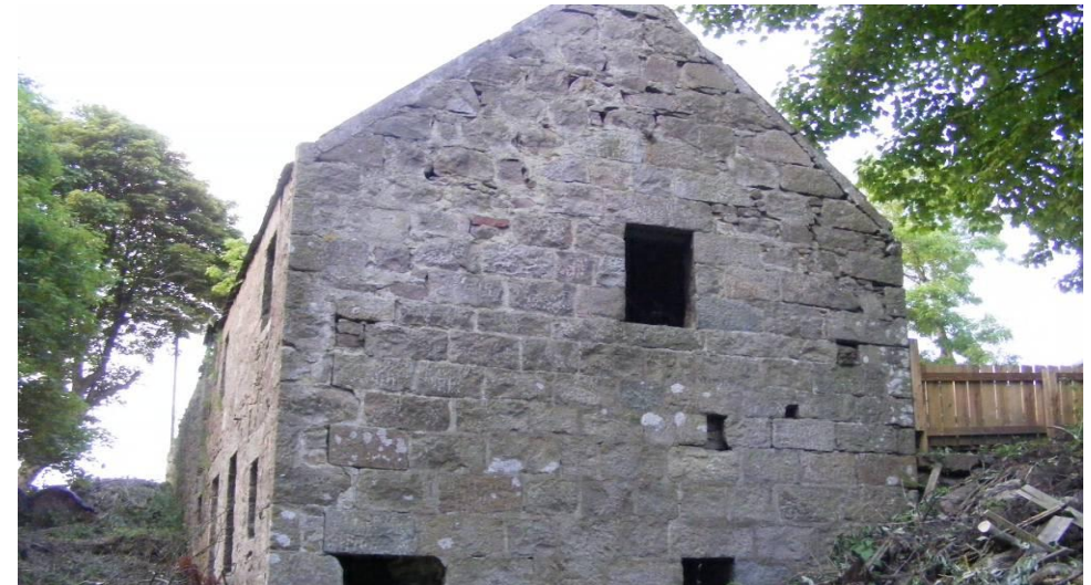
Photo 7: South elevation of mill. Some large holes in wall which had some cracks, however, no evidence of bats were found. Small, shallow cracks near top of mill could provide limited roosting potential. No evidence of bats was found.
