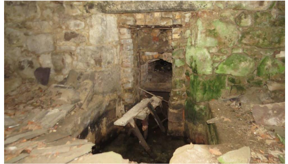
Photo 14: Lower floor, north gable of main building. Grain drying kiln floor has fallen in. The walls are damp and have no cracks. The grain kiln has a collapsed chimney. Inspection showed no evidence of bats
