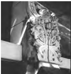
Typical bad repair
