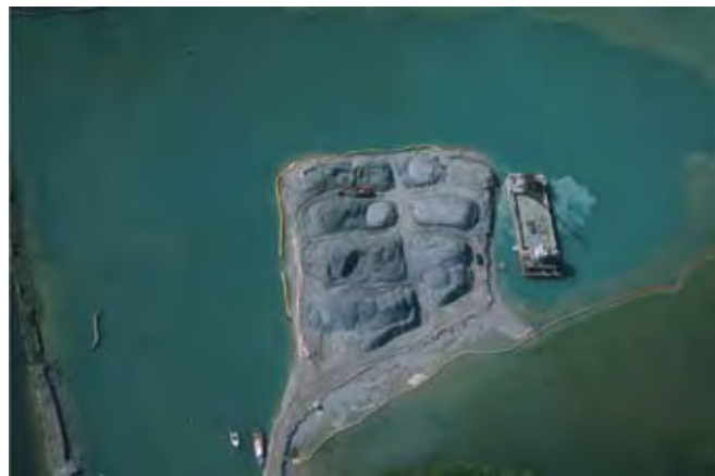
Figure 15.3 At Imul village in Aimeliik State, an area of shallow flats adjacent to an existing dock and abutting a deeper channel was dredged for Compact Road fill. A barge-based crane removed the fill and deposited it onshore, in a storage area, so that it could drain. Trucks picked up the material and took it to the worksites from the storage area. The dredging area was surrounded by a silt fence. The operation has now ceased, leaving a deep sediment bottom area connecting with a channel giving boat access to the dock. This area is also shown in a wider view in Figure 14.6a.
