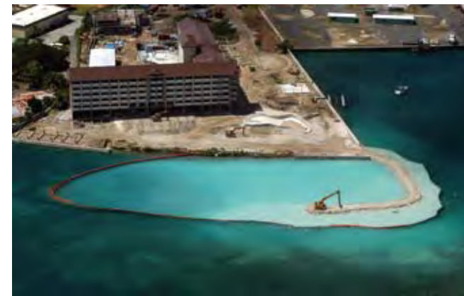
Figure 15.7 As part of the development of the Palau Royal Resort on Malakal Island in 2004, a new boat channel was dredged along the shore of the resort. The work was done by a mechanical excavator working along a berm extending from the shore as well as directly from the shore. This produced a deep boat channel right along the nominal beach of the resort. In 2007 it was decided that a real beach was needed, so a new channel was dug and the area dredged in 2004 was filled to produce a beach and swimming area. A silt curtain reduces the amount of fine suspended sediment emanating from the site, but is far from faultless. Small amounts of sediment-laden water get around the curtain, particularly as the 2 m tide falls, forming a plume of milky water. If this project had been well-thought-out and done correctly from the start, much potential damage to the marine environment could have been prevented.
