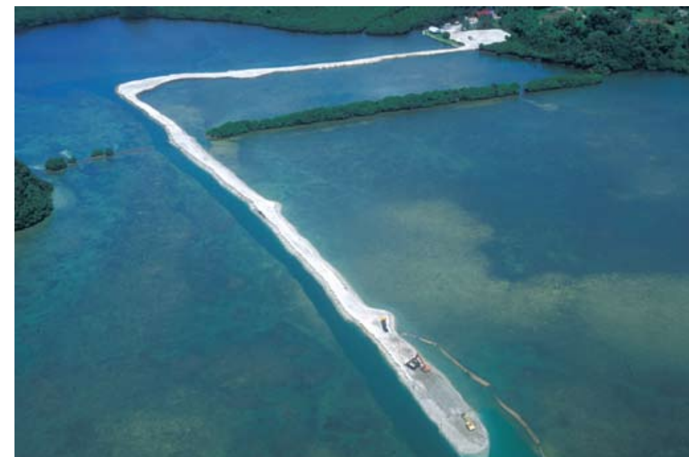
Figure 15.1 Dredging activities are occurring in many areas of Palau for a variety of reasons. A photo taken off Airai village shows a small boat channel being dug across a wide expanse of shallow flat. The channel is excavated through construction of a temporary berm beside it. A self-propelled excavator starts from shore and moves onto the flat, digging the channel and depositing the spoil alongside the channel. This then makes an above-water road which the excavator can use to go out further onto the flat, alternately digging the channel and building the berm. If the bottom is shallow, the berm, as seen in this photo, can be quite long. At the end of the process, the berm material can either be left in place (where it can possibly wash back into the channel) as a breakwater, or it can be hauled away in trucks for use as fill elsewhere. The material generated by this project is destined for fill, although as of 2007 only the outer part of the berm has been removed. This particular channel had to be sharply angled and made much longer than absolutely necessary, because it had to go around a Japanese era stone breakwater built across a gap about half a km wide.
