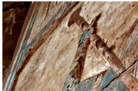
Fig. 9.84: Line of roughly cut back stone along the top edge and side of the bas-relief with the poor quality of the finish and lack of decoration.
