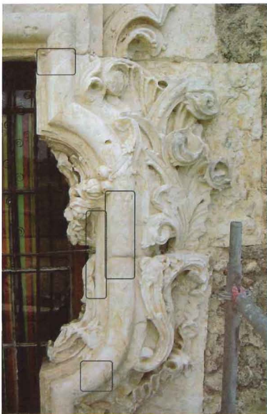
Fig. 9. The outlined areas are finished mortar fills that replaced incompatible previous repairs.
