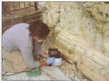
Fig. 6. Preconsolidation of the Sacristy Window limestone with HCT applied in a power sprayer.
