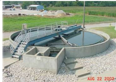
A circular settling tank
