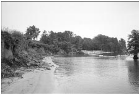
Figure 112: Shore Erosion at Governor's Land on the Chickahominy River, Virginia, 1990. (Photograph courtesy of the National Park Service)
