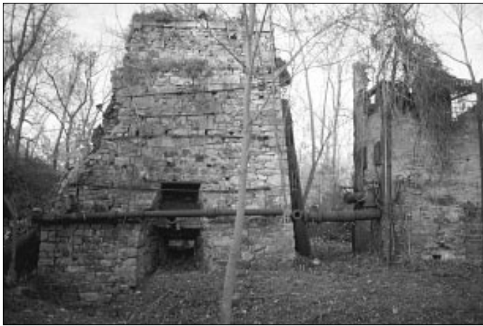
Figure 26: Fragment of an Industrial Landscape: The smelting stack at Principio Iron Furnace, Havre de Grace, Maryland, in 1997. (Photograph courtesy of the National Park Service)
