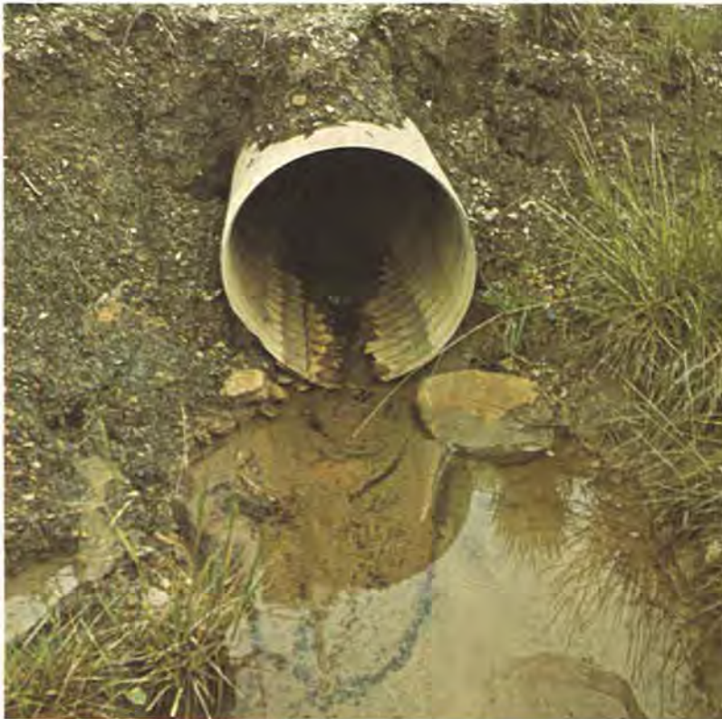
An Example of the Corrosive Nature of Mine Drainage.
