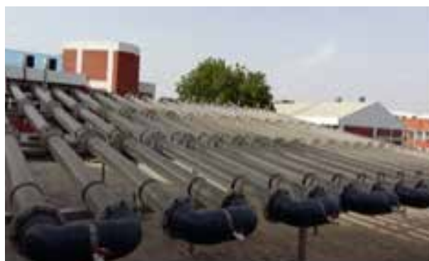
3000 litre Tubular Algae Photo Bioreactor facility at DBT-IOC Center Faridabad
