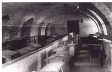
In this women's balcony in Slonim, the rounded ceiling gives a prayerhouse atmosphere. Windows at the right are for sunlight. Those at the left face down onto the main area of the synagogue.
