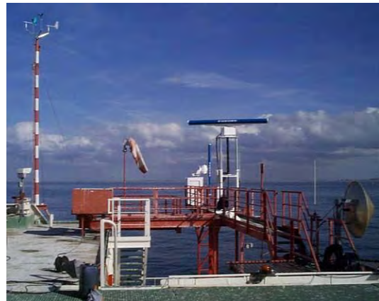
MERLIN system HSR (foreground) and VSR (rear) installation on Meetpost research platform (2003)
