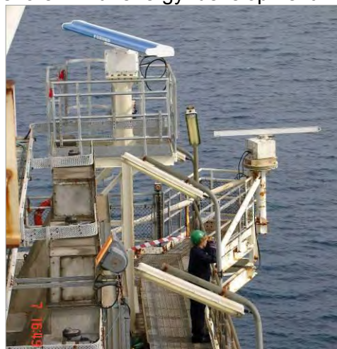
Furuno marine radar on the Talisman-Beatrice platform (top unit - blue); the MERLIN processor was installed in the equipment console to the left.
