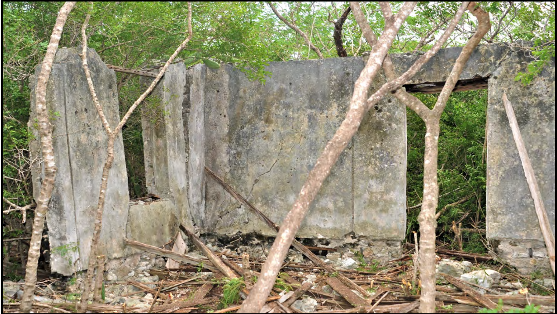
Plate 10. Structure 5. Interior view of southwest corner showing dangerous structural disassociation. Narrow vertical grooves in plaster represent otherwise lost timber internal partitions.
