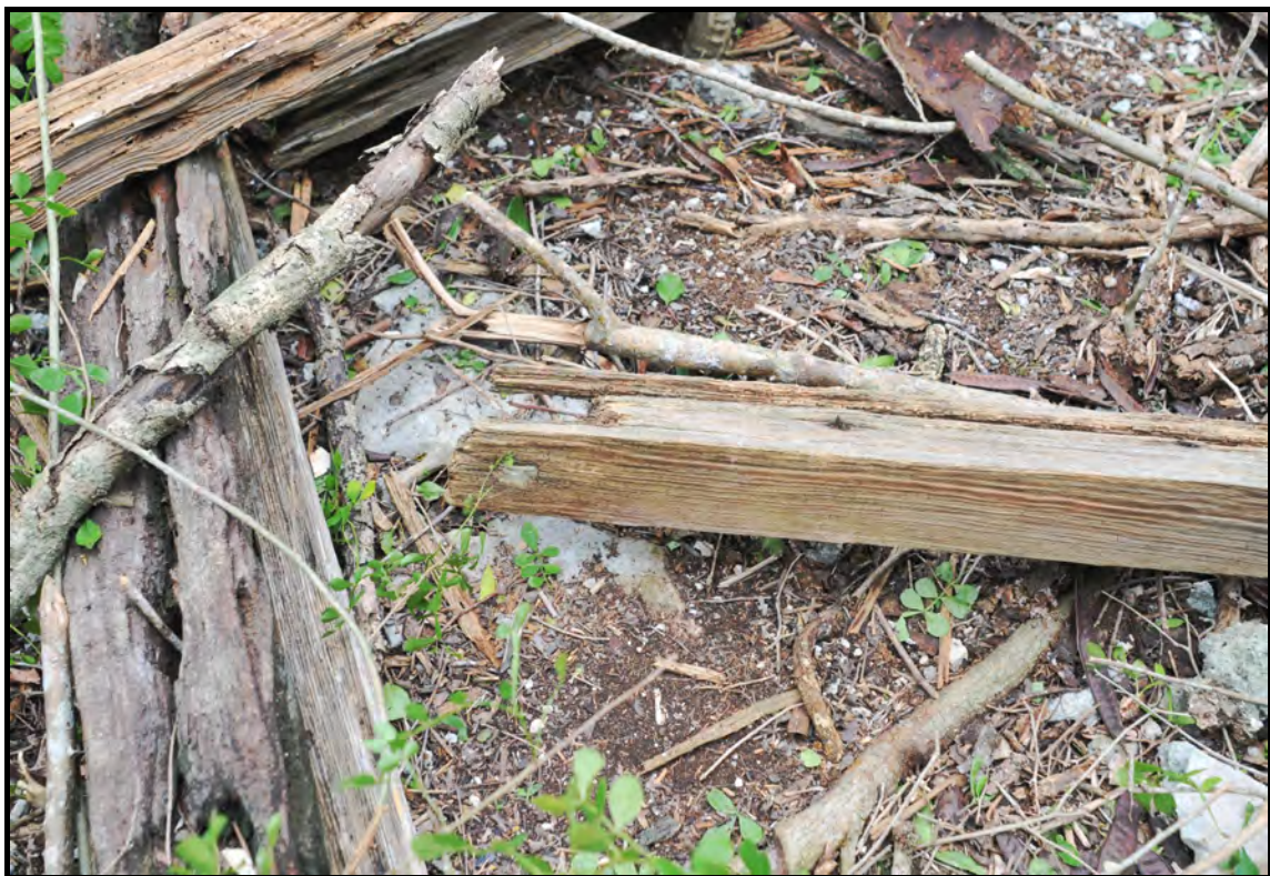
Plate 3b. Structure 1, roof framing, detail of fallen ridge rafter.
