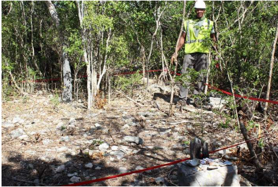
Fig.6 Red survey tape outlines wooden post holes cut into the bedrock for a wood-frame building.
