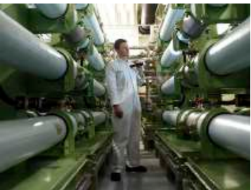
All Disney Cruise Line ships are equipped with Advanced Wastewater Purification Systems.
