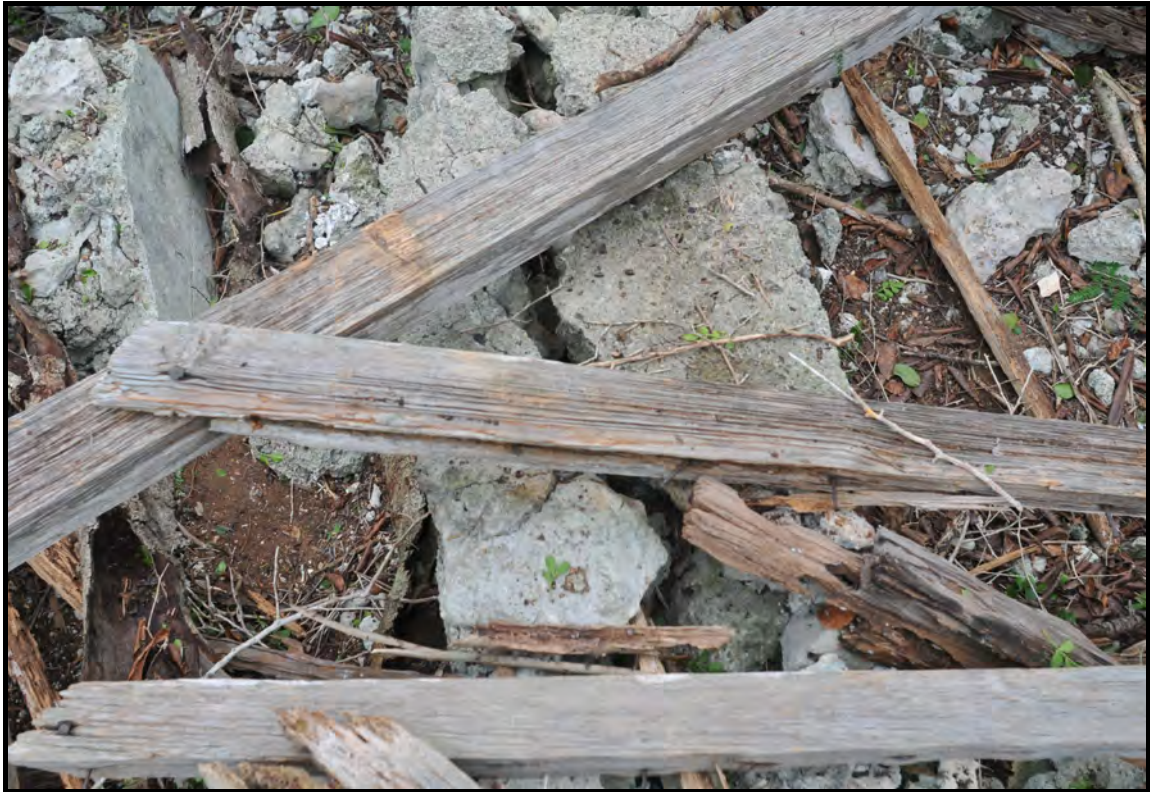
Plate 3a. Structure 1, roof framing, detail of fallen rafters
