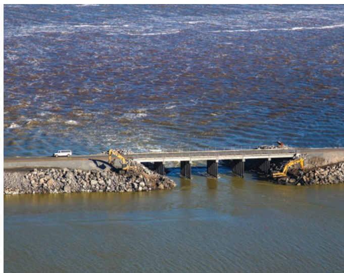
On 12/1/16, the Union Pacific Causeway was breached as part of an agreement, brokered by the Council, to help balance salinity levels in the North and South arms. A control berm will facilitate adaptive management. Elevation equilibrium will likely be reached next fall. © Wayne Wurtsbaugh, LimnoVision, pilot: Tom Rollins.
