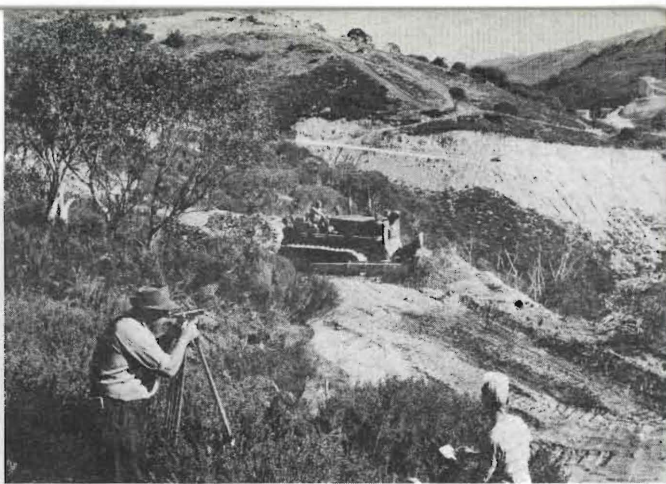
Surveying for a new road which will form part of the Snowy Mountains Scheme.
