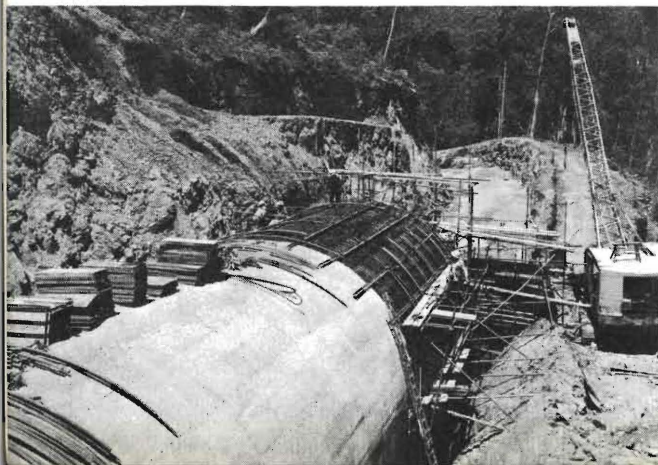
Construction of an underpass to take a road beneath the Murray No. 1 pressure pipelines.
