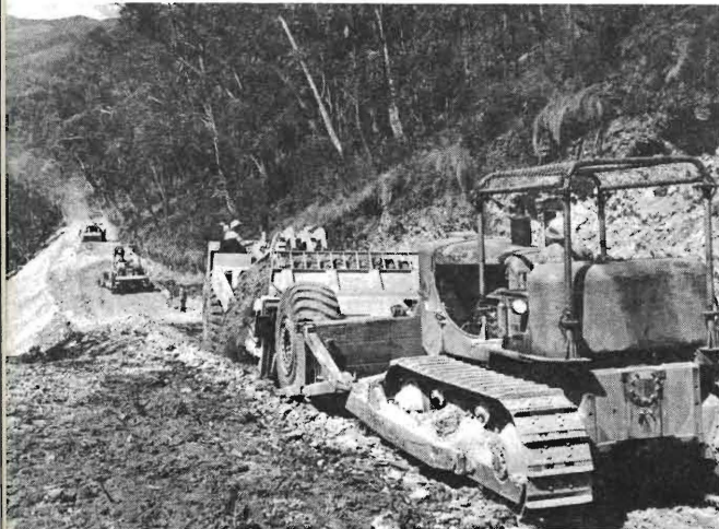
Heavy earthmoving and road construction equipment cutting an access road through to the new Murray No. 1 project in the Snowy Mountains.
