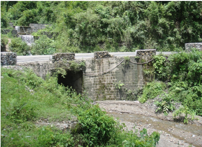
Vegetation and pipe that could be damaged
