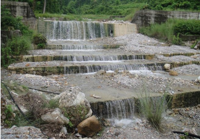
Check dam has to be improved.
