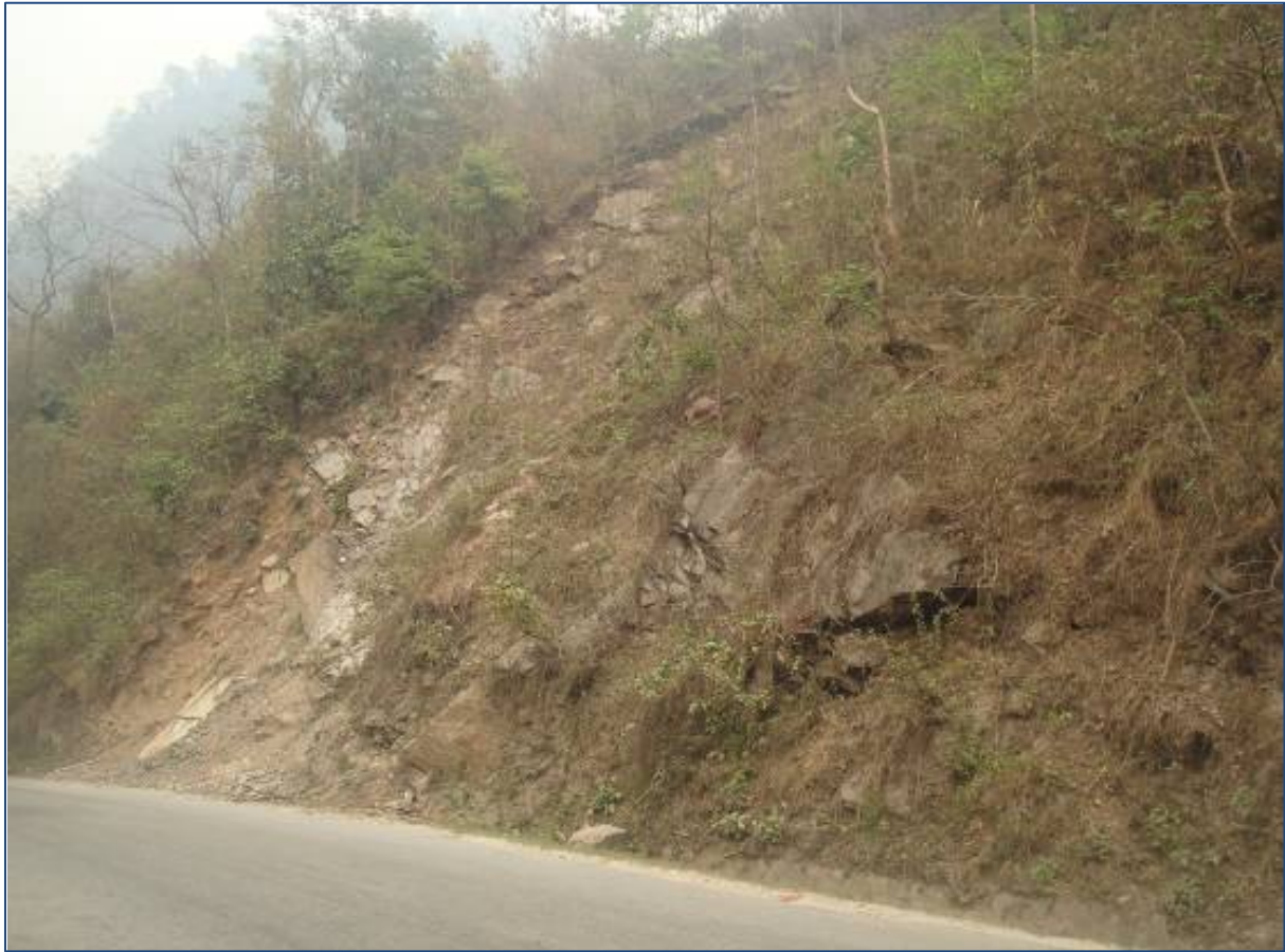
Photo 4.3 : Existing Landslide at Km 17 +800
