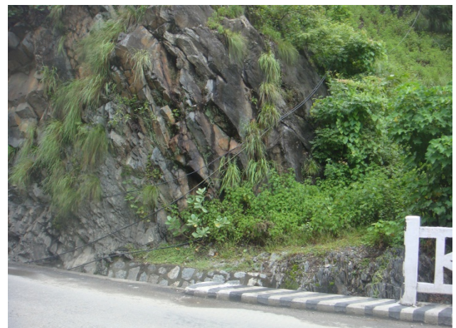
Water pipe line that could be damaged
