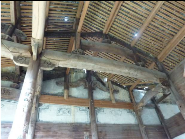
General Ancestral Temple of Yu's Ancestral Temple in Qingxi Village – Wooden Structure
