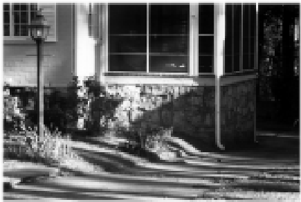
This granite foundation is characteristic of houses found in Emory Grove and should be properly maintained
