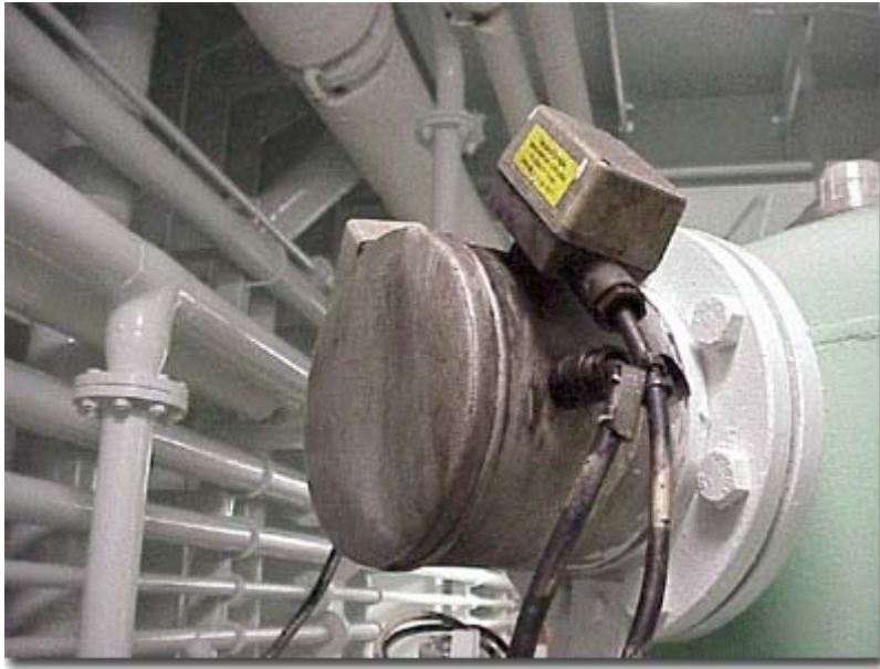
Εικόνα γ61 : Oil filtering equipment monitoring and control system
