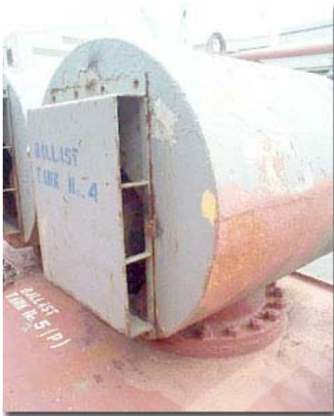
Εικόνα γ36: Ball-type ballast tank ventilators headed with wasted inner/outer wall(1)
