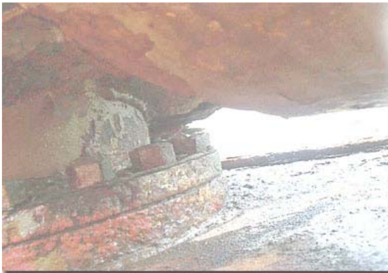
Εικόνα γ37: Ball-type ballast tank ventilators headed with wasted inner/outer wall(2)
