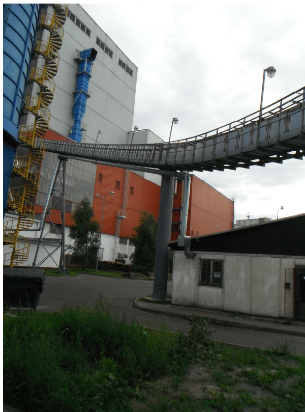
Obr. 12 Samostatná trasa peletek do kotle K4, K5
