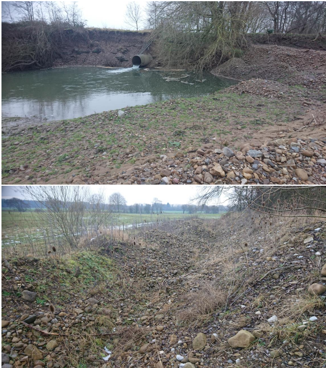
Fig 17b. Upper: the 'confluence' of Fiddale Beck with the Swale, piped unceremoniously through a perched culvert. There was evidence of recent and ongoing plant activity shifting substrate around , presumably in a futile attempt to protect the culvert pipe environs.
