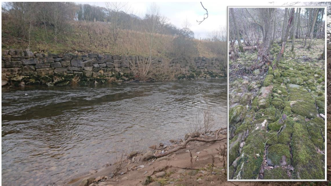
Fig 5. A highly engineered solution of boulder revetment / walling to the LB to prevent the river returning to a natural course u/s of Abbey Farm (Easby Abbey Mill). It is unclear how long ago the weir (shallow, dressed stone; inset) that fed the mill failed, but the increased gradient at this point probably contributed to the excessive erosion.
