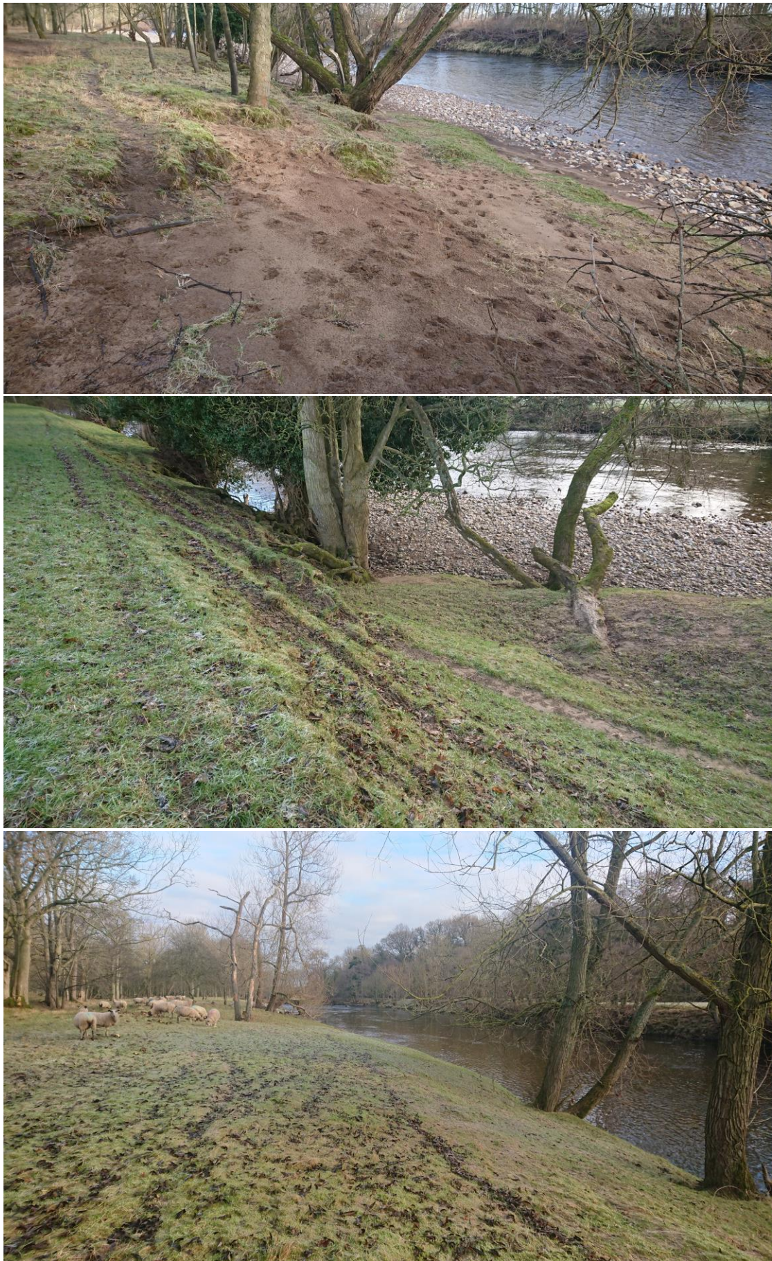
Fig 13. There was plenty of evidence of the damage that sheep can do to river banks which leaves the friable soils more susceptible to erosion: continued disturbance of unconsolidated material (upper); desire line tracks weakening the integrity of the soil (mid); and maintenance of short sward grass with poor root systems (lower).
