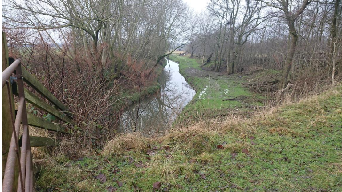
Fig 18. Looking upstream along the straightened and dredged channel of Fiddale Beck from the vantage point on top of the Swale flood bund and almost directly over the top of the culvert that links the two.
