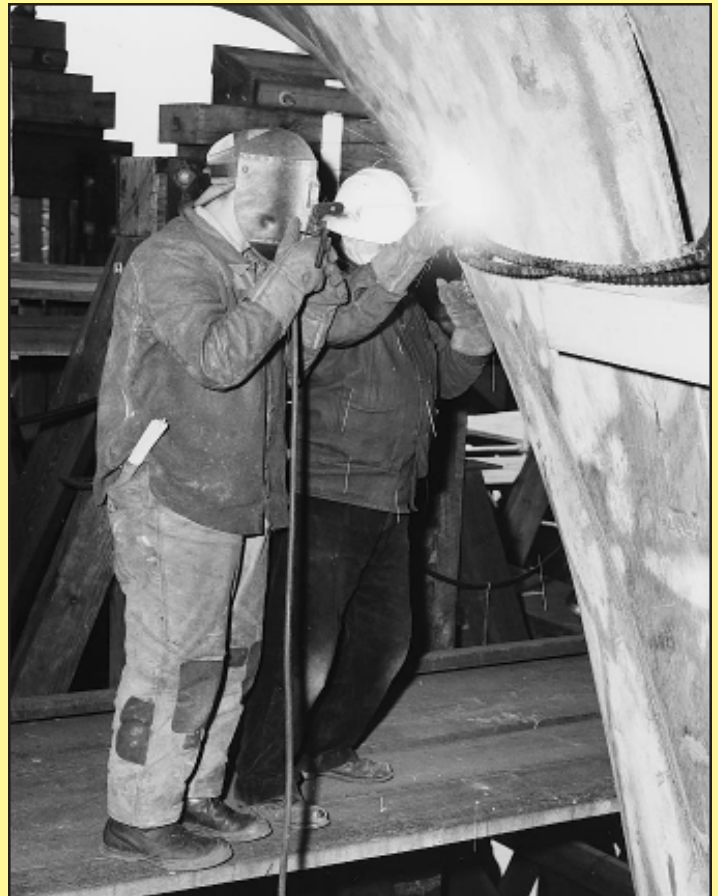
WELDER — As all-welded hulls replaced riveted hulls, the welder assumed greater importance in the yard. Here a welder works on the construction of USS Suffolk County (LST-1173) in early 1956. BOSTS-14320
