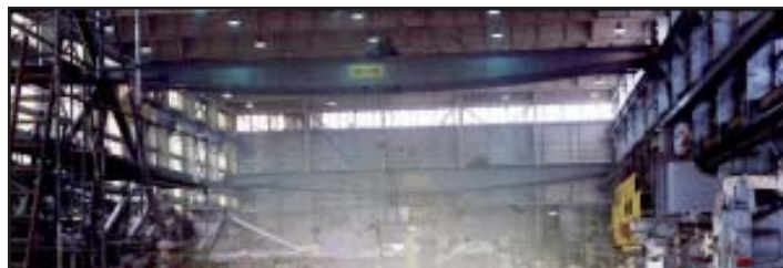
BRIDGE CRANE — Bridge cranes served most of the industrial buildings in the Navy Yard, allowing heavy materials to be moved throughout the length and width of their central bays. This pair of 5-ton capacity cranes is in the Structural Shop in the Building 104 Extension. Note how they are on different levels so they can pass each other. BOSTS-15920
