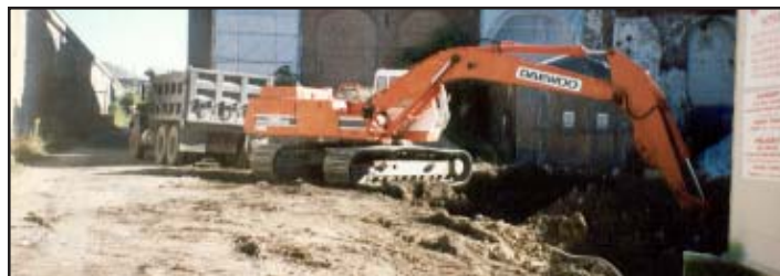
In 1994 the U.S. Army Corps of Engineers removed the underground fuel tanks outside of the Power Plant (Building 108) in the Navy Yard. Two years later, the Corps returned to the site to ensure that all contaminated soil in the area had been removed. U.S. Army Corps of Engineers
