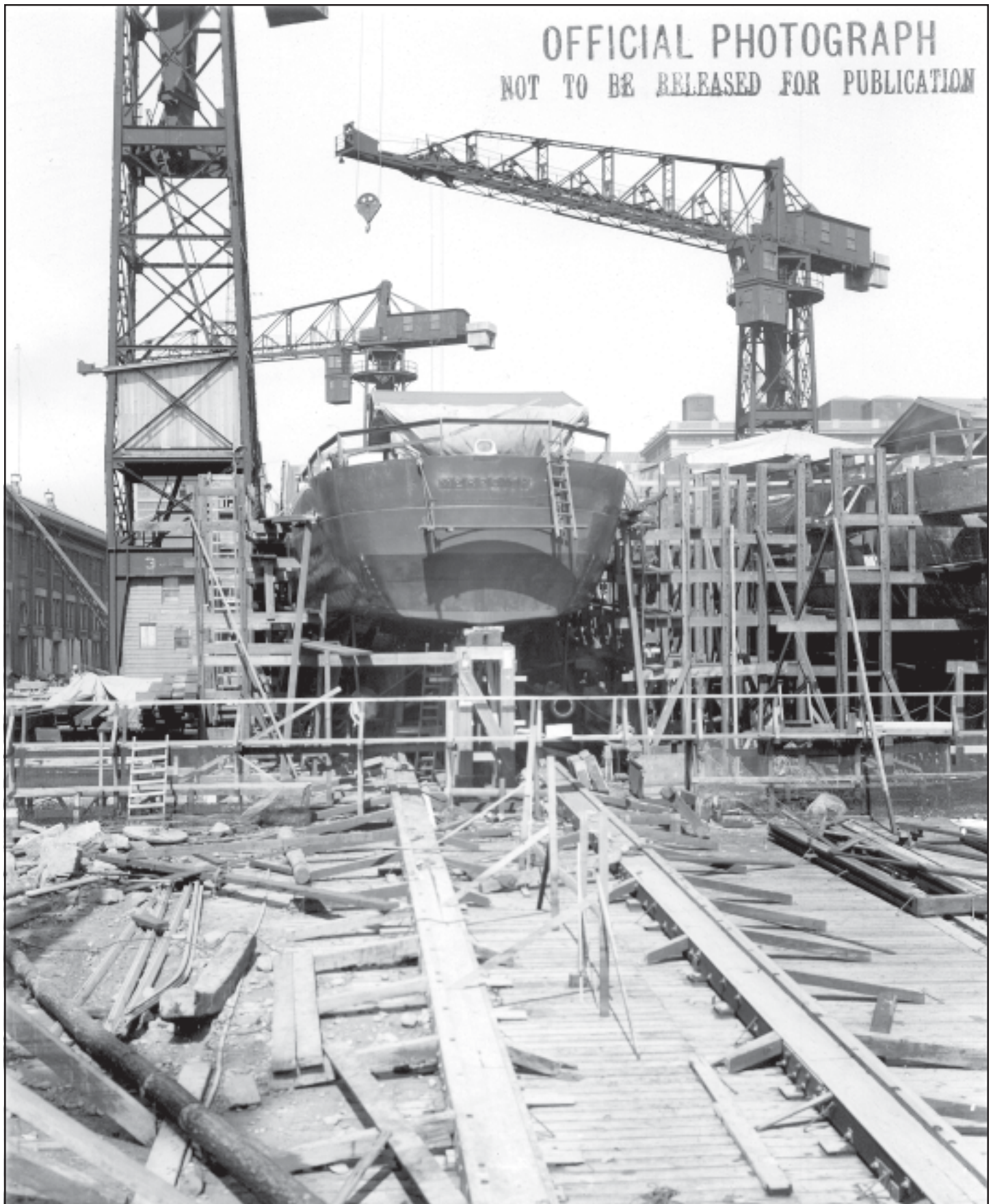
The peak period of shipbuilding at the Charlestown Navy Yard came immediately prior to and during World War II. This Apr. 1, 1940, image shows the destroyer USS Meredith (DD-434) under construction on Shipways 1. She would be launched a little over three weeks later, on Apr. 24, 1940. A sister ship, USS Gwin (DD-433), can be seen to her right. BOSTS-11972
