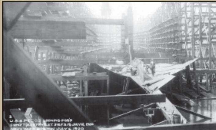
A little over a month later, on July 6, 1920, the bottom of the vessel was beginning to take shape.
