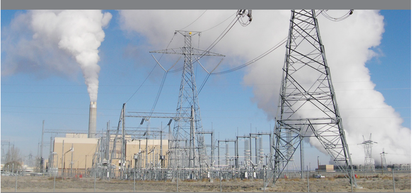
Electrical transmission lines at the IPP coal plant, Utah. Photo Credit: Michael Vanden Berg, UGS
