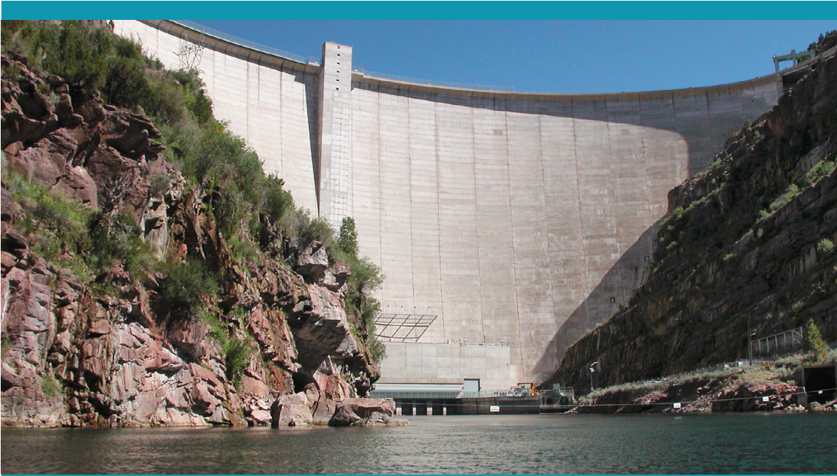
Flaming Gorge Dam, Utah. Photo Credit: Michael Vanden Berg, Utah Geological Survey
