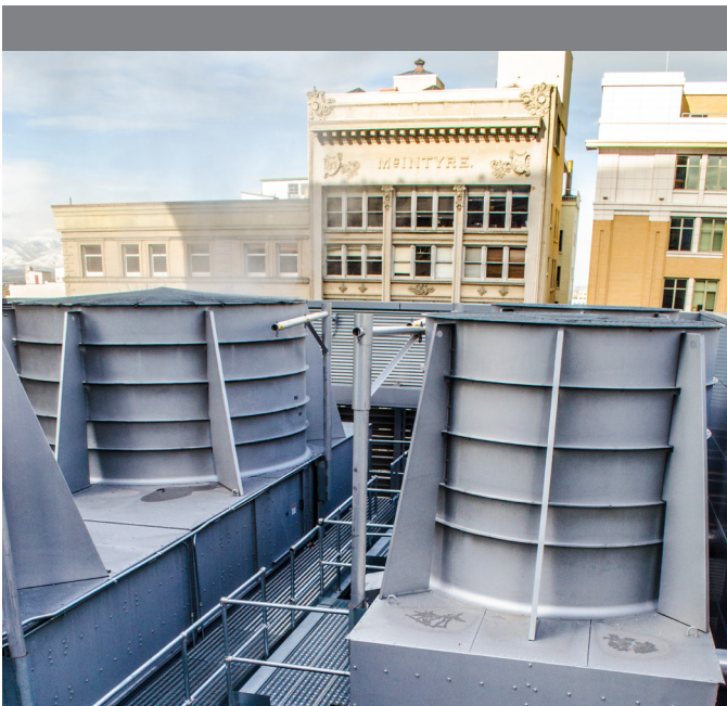
Cooling towers in the City Creek development in downtown Salt Lake City utilize some of the most energy efficient technologies. Photo Credit: Andrew Gillman
