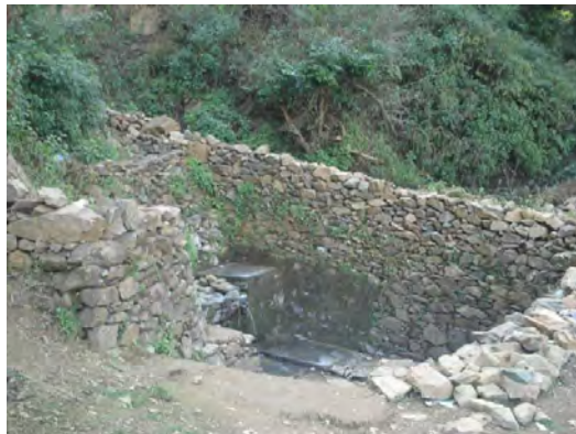
How long will this survive: A spring by the side of this excavation, the terraced fields are already short on irrigation infrastructure
