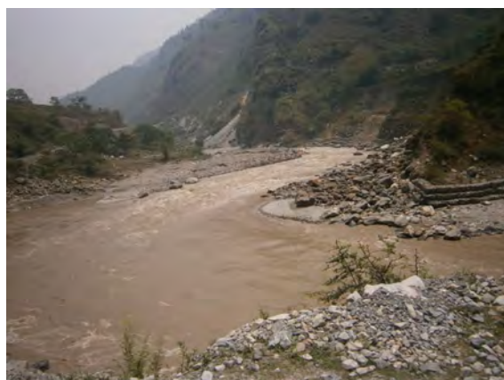
A sharp meander near Kalika, a few meters upstream the road was washed away in 2016
