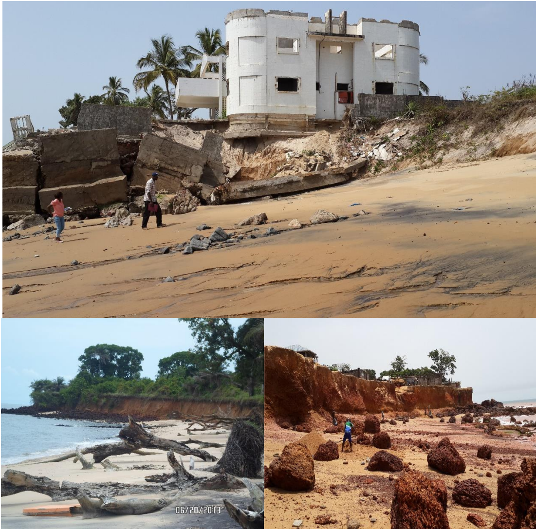
Coastal Erosion in Lakka, Shenge and Hamilton
